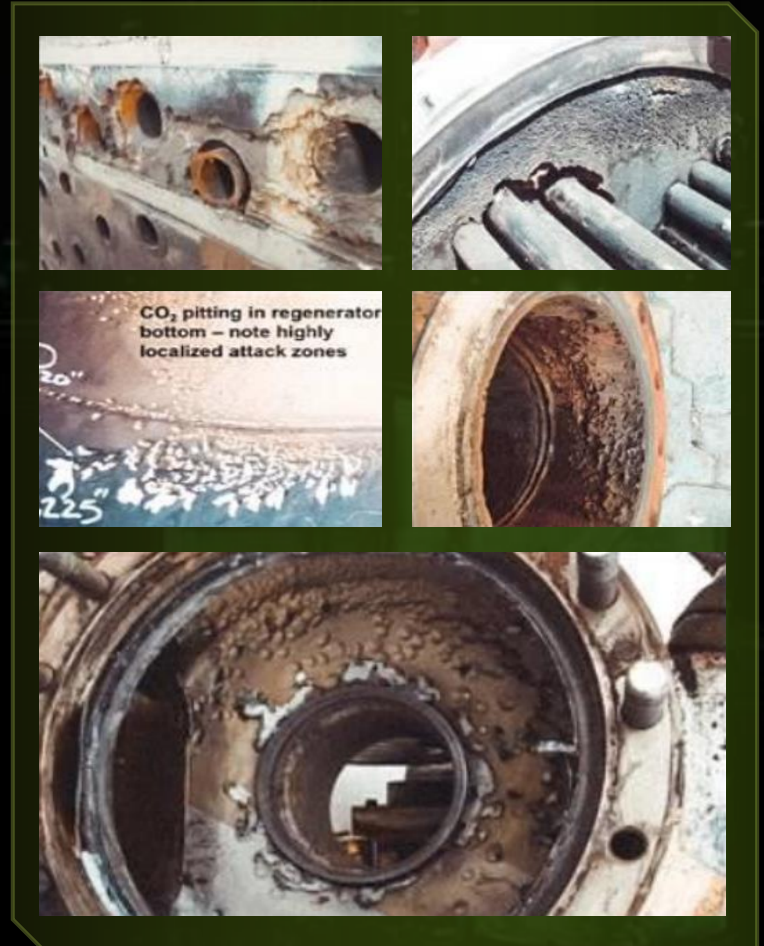
Examples of Corrosion Caused by Excessive CO 2 in Various Locations of an Amine Unit
